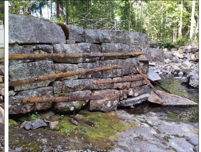
Figure 17. Example of hard bank protection. Note breached section on right side of photograph.
