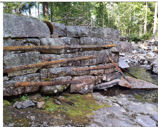
Figure 17. Example of hard bank protection. Note breached section on right side of photograph.
